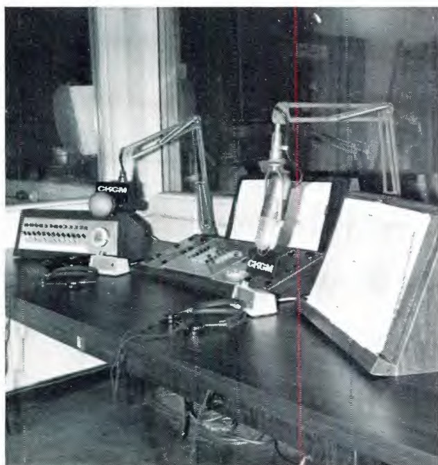
Fig. 6. ON AIR studio arrangement shows all components.
